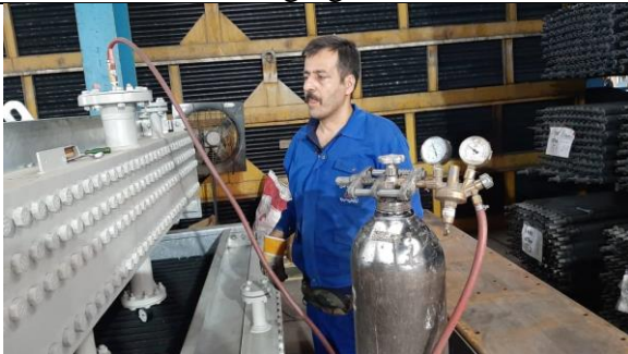
N2 Purging control
