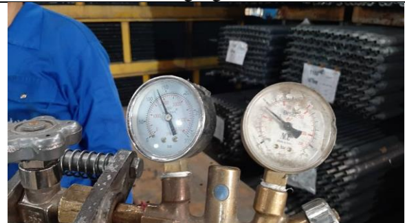
N2 Purging control
