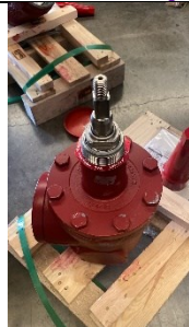
Inspection of 2nd Compressor - Spares
