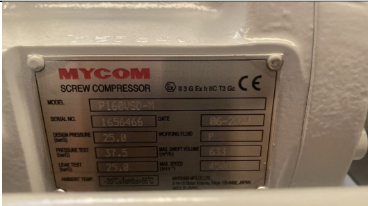
Inspection of 2nd Compressor Skid
